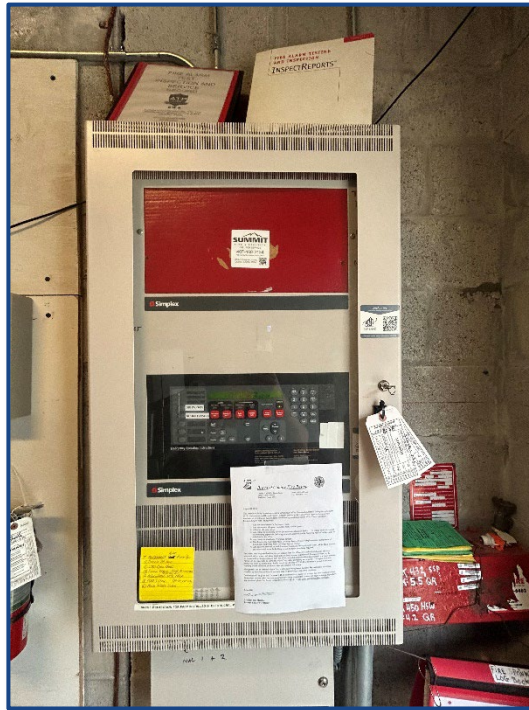
Photograph No. 23: Simplex Fire Alarm control panel located in the utility room.
