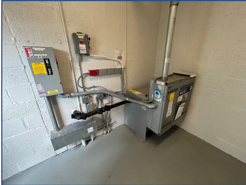
Photograph No. 24: Typical elevator hydraulic unit in the utility room.
