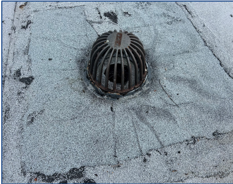
Photograph No. 14: Typical interior roof drain at the center of the roof.
