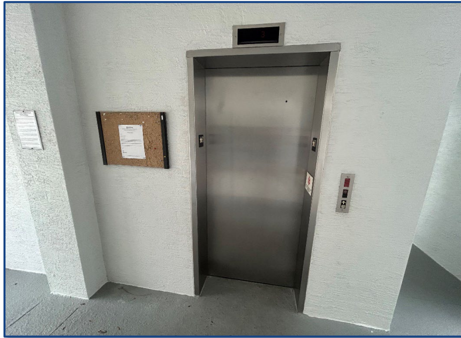
Photograph No. 21: Typical elevator door at center of building.
