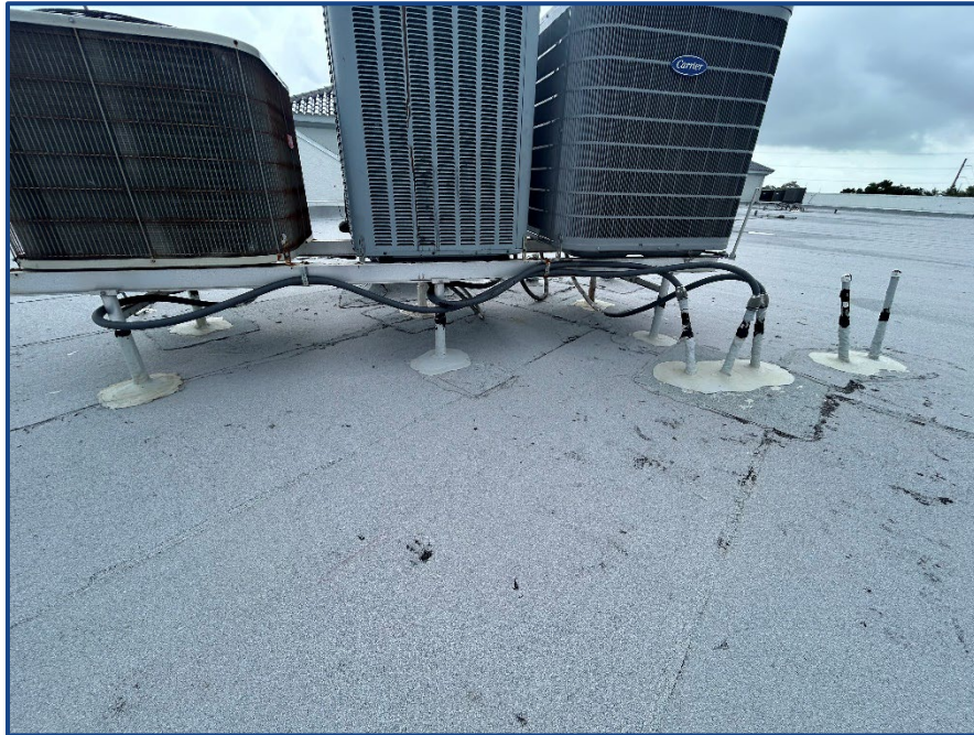
Photograph No. 16: AC stands mineral covered supports.
