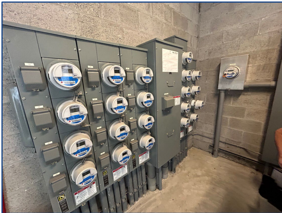
Photograph No. 22: Typical electrical meters and main service panel.
