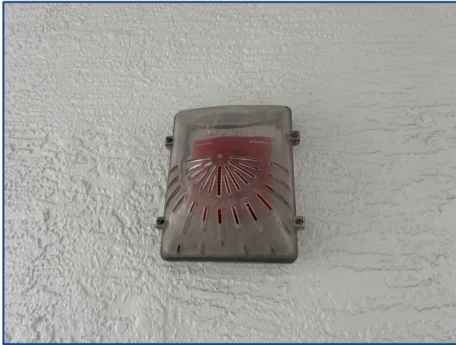
Photograph No. 27: Typical fire alarm located in walkway.
