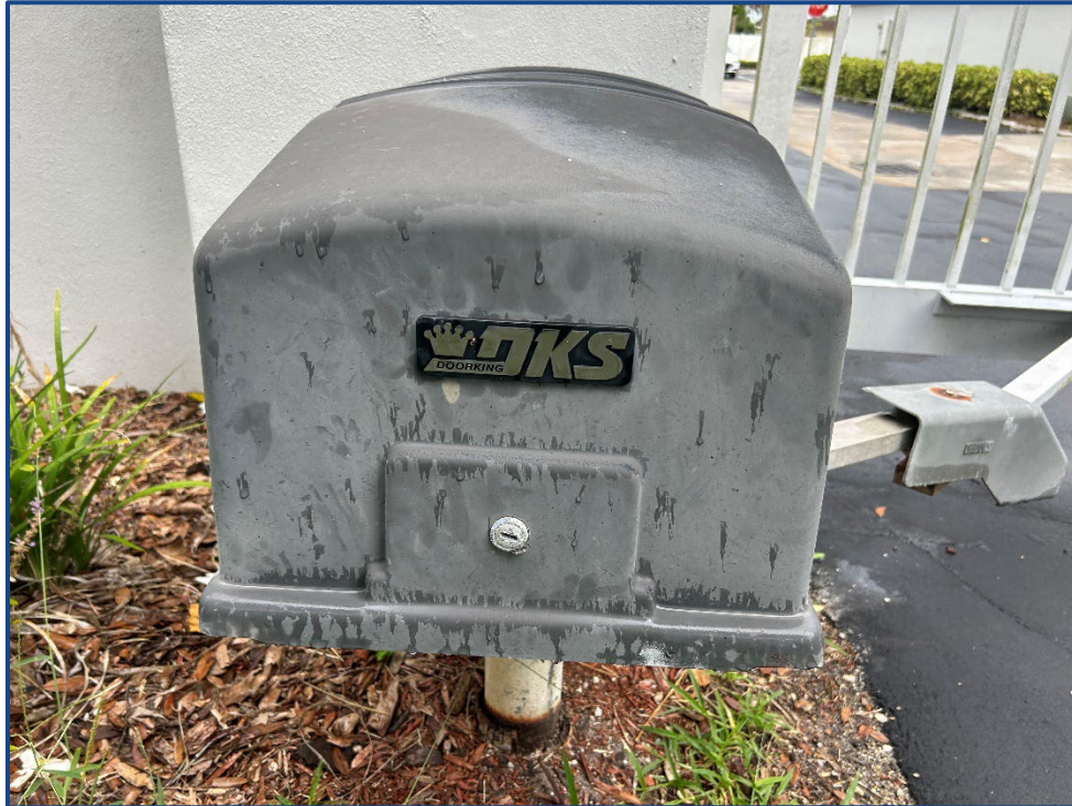
Photograph No. 28: Entrance gate motor at the south side of the property.
